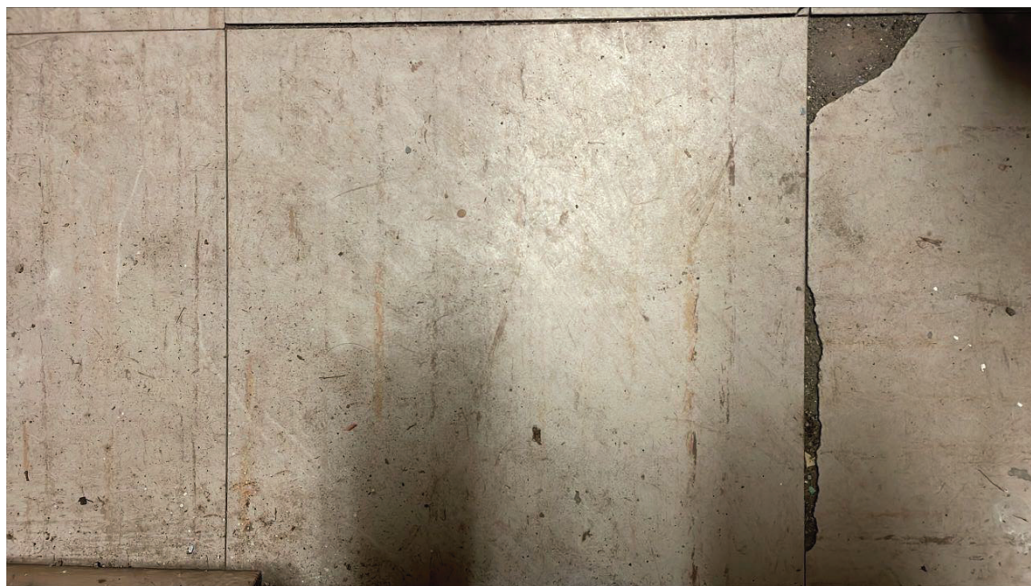
Figure 1: Asbestos-containing 12"x 12" vinyl tile from Basement
