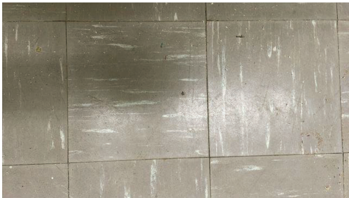
Figure 3: Asbestos-containing grey 9"x 9" vinyl tile from Carpentry Shop
